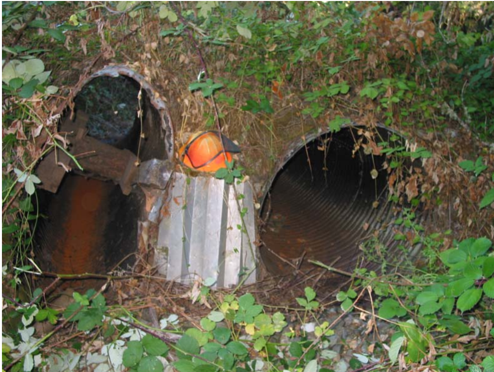
Figure 24. Culvert #2 inlet on Jordan Creek at north end of Rod & Gun Club Road.
