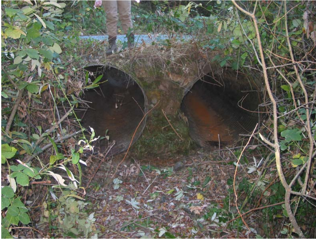
Figure 23. Culvert #2 outlet on Jordan Creek at north end of Rod & Gun Club Road.
