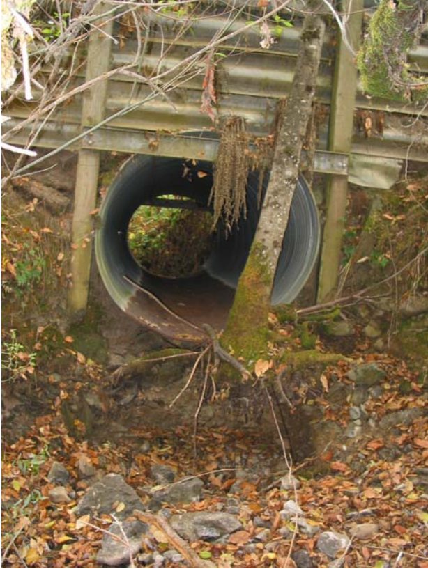
Figure 27. Culvert #5 outlet on Jordan Creek at driveway off Rod & Gun Club Road.
