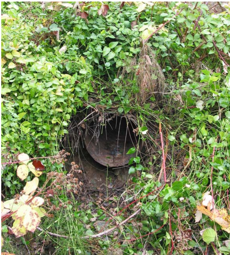
Figure 26. Culvert #4 outlet on Jordan Creek at washed-out road off Rod & Gun Club Road.
